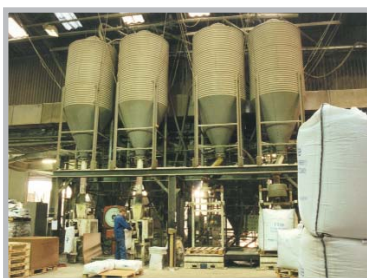
Filling materials in Bulk Bags and 50lb bags in a minerals processing plant.
