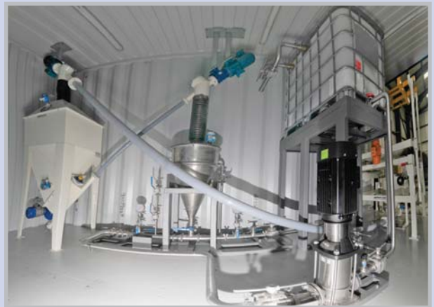
Water treatment system inside an ISO container
