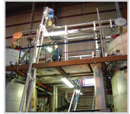
Inclined & horizontal AMCs feed additives to either of two (2) tanks.
