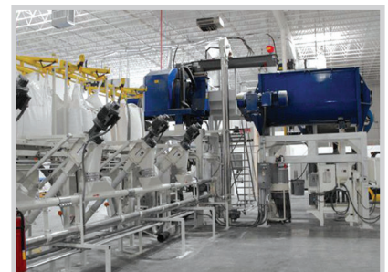
An AMC with multiple inlets delivers cement, sand, ash & recycled glass to a second unit that lifts them up into a mixer.
