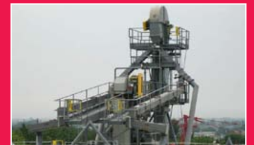
Two bucket elevators transfer fly ash from rail receiving into bulk storage tanks.
