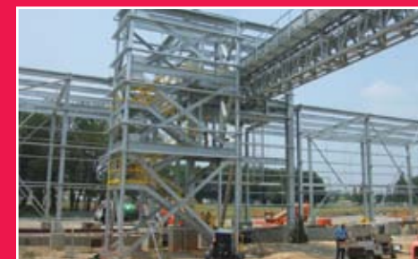
This transfer tower and enclosed trussed conveyor are designed to move product from bulk storage to processing.
