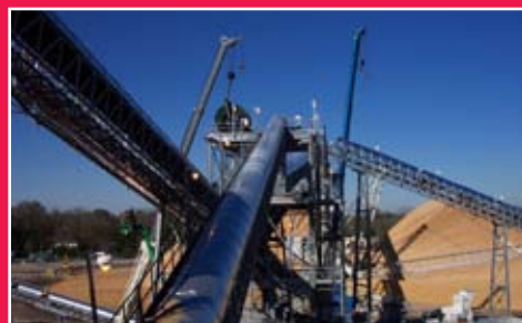
Trussed transfer conveyors move raw material to and from bulk storage.
