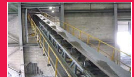
Our trussed CTR conveyor is shown taking product to truck load-out.
