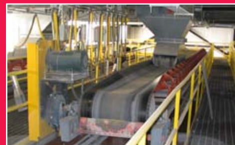
A reversing and shuttling conveyor transfers a sticky clay material into one of several storage tanks.
