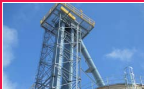
A bucket elevator is shown filling limestone into a large industrial storage silo.
