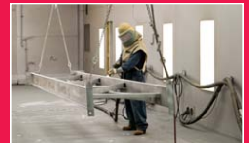
Quality paint starts with superior finishing equipment. We have a wash bay, sandblast booth, a wet enamel booth and a state-of-the-art powder coat system.
